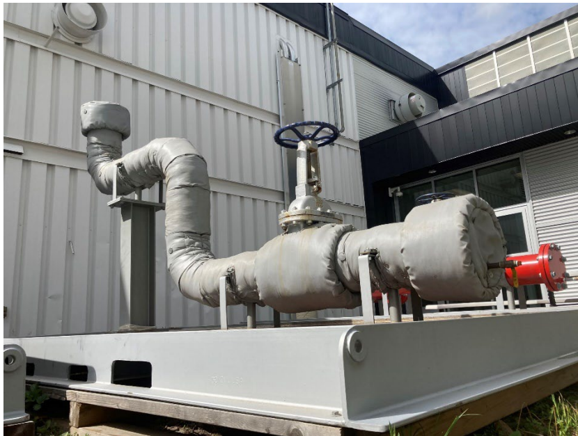
Figure 6: Copper-nickel seawater cooling pipe test panel. Large circular defects representing general corrosion and small blind holes representing pitting corrosion were machined into the inner surfaces of the pipe at depths ranging from 10 to 50% of the pipe wall thickness. The entire pipe was wrapped in 1" thick insulation which could not be removed for inspections. Photo credit: Centre de Métallurgie du Québec.
